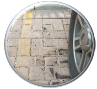
Permeable pavers are a BMP
