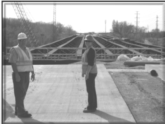
Pat Kelsey, WBK and Resource Analyst Candice Jacobs during weekly Stearns Road Bridge Inspection
